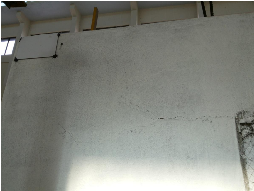
Fig. 37 Cracks in the eastern wall at the top level near door opening
