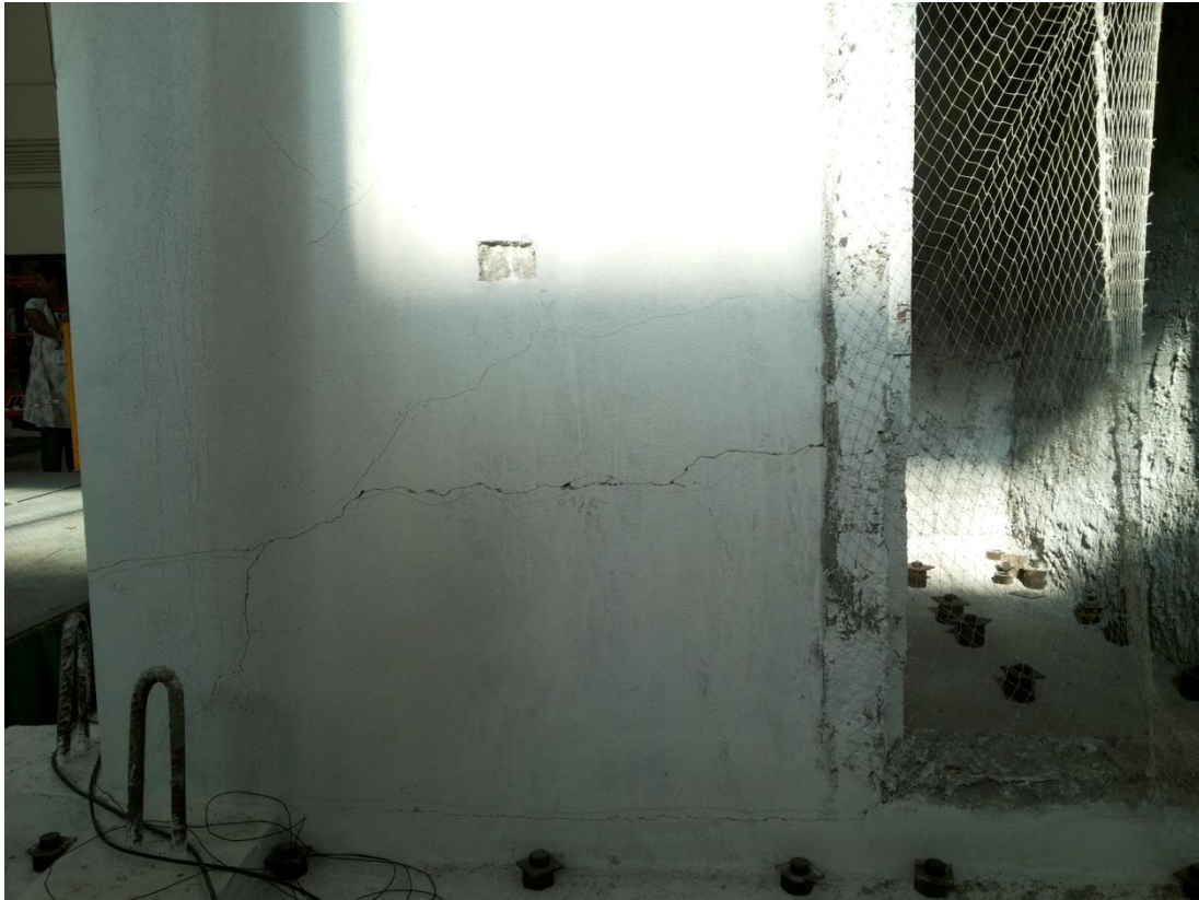
Fig. 36 Cracks at the bottom level in the eastern wall with door opening
