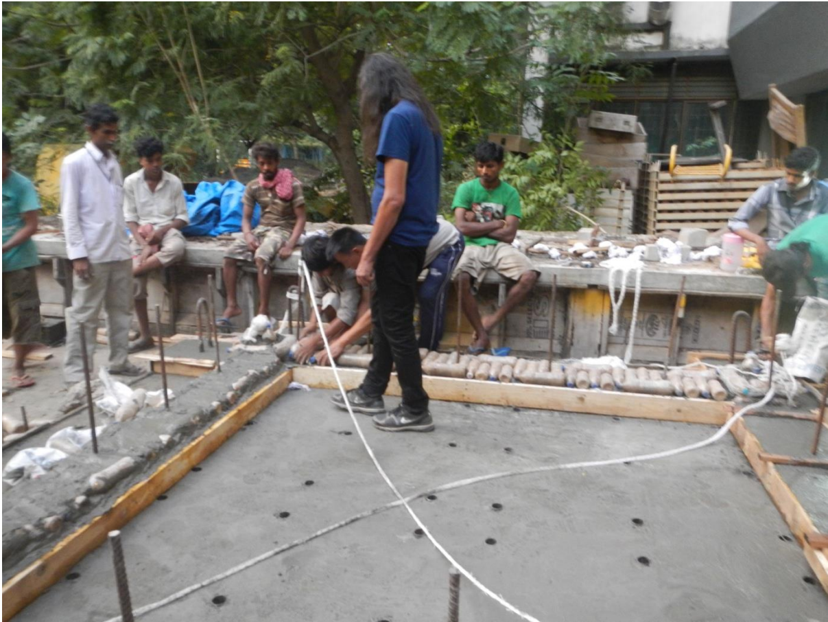
Fig. 7 First layer of PET bottle walls laid using horizontal staggered bottles on fresh concrete
