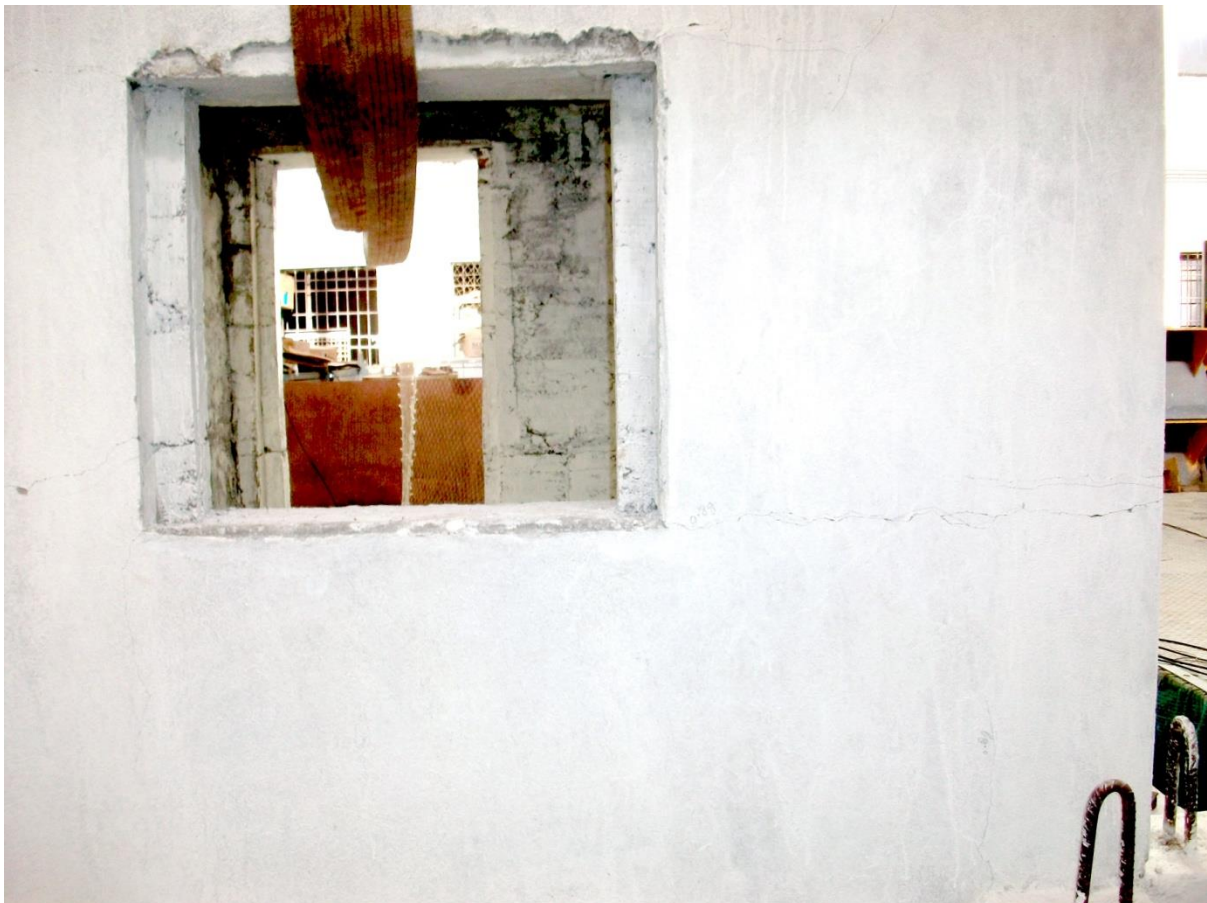
Fig. 31 Cracks observed in the western wall (with window opening)
