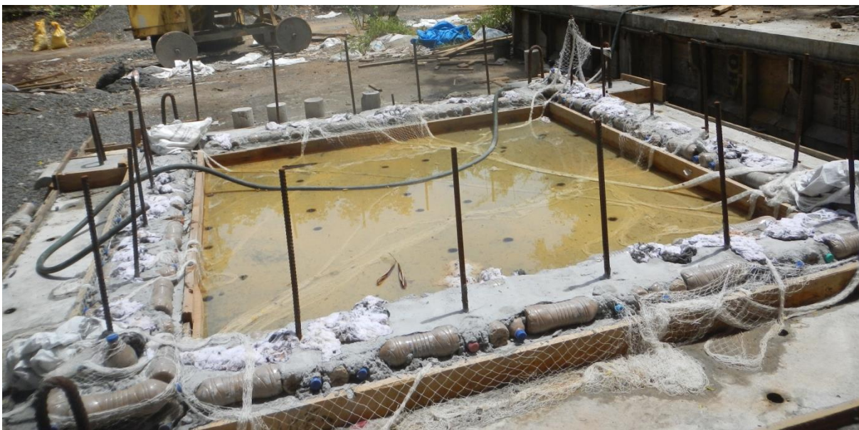
Fig.8 Finished RCC slab with one layer of PET bottle walls and columns under curing
