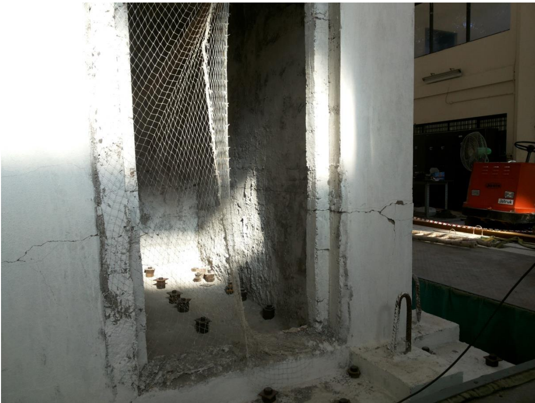
Fig. 35 Cracks in the eastern wall with door opening
