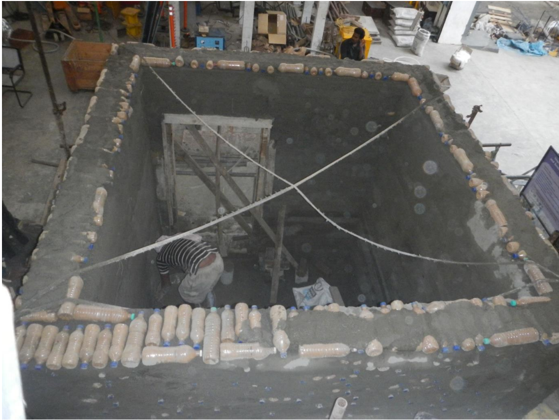
Fig. 13. Top view of the finished structure with fishnets across the roof slab.
