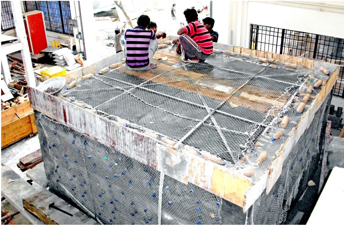
Fig. 14. View of the fishnets across the roof slab.
