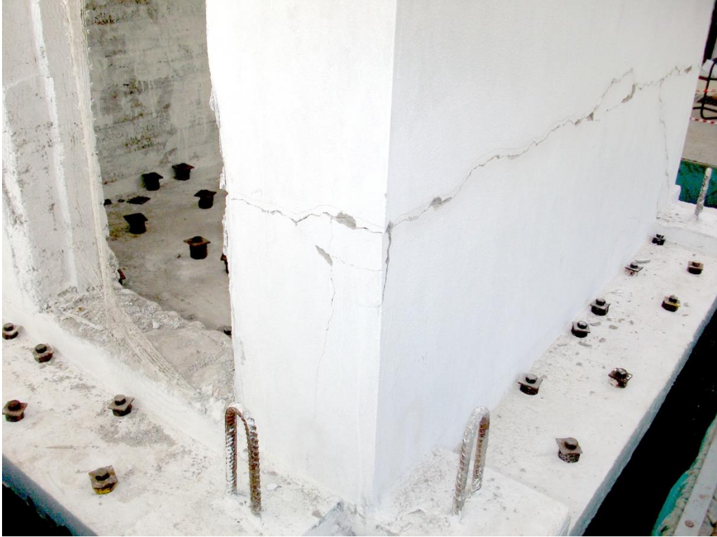
Fig. 34 Failure cracks in the north eastern corner
